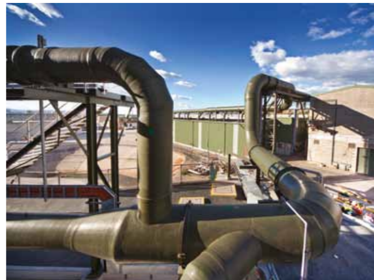
Top left and bottom - Odour Control Facility (Wollongong, NSW): Demolition of old and construction of new odour control facility and extension of biosolids room including earthworks and structural works. Abergeldie designed, fabricated and installed all FRP ductwork and nutrient transfer, storage and dosage systems.
