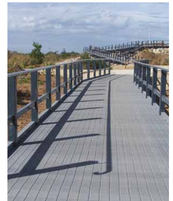
Blue Water Trail (Mackay, QLD): Completed for Mackay City Council as a means to improve community well being and recreational opportunities. Abergeldie constructed 1km of raised boardwalk above environmentally sensitive wetlands and a 30m bridge over Alligator Creek. The scope also included installation of 1.2km of footpath, fencing, landscaping, street lighting and furniture and a car park.
